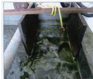
图5 翻滚的腐蚀液 Fig.5 Rolling corrosion liquid
